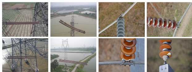
(a)正常 (b)掉串 (c)破损 (d)闪络
